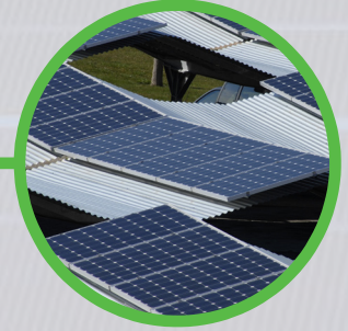
MARQUESINAS. 63 kWp Paneles monocristalinos Parking lot roof Monocrystalline cells
