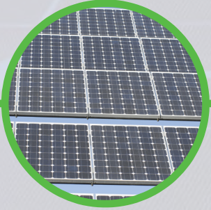
MECASOLAR. 10,6 kWp Panel union heterogénea Multi-junction cells
